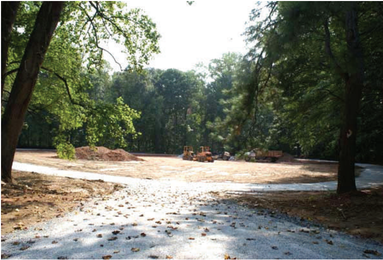
Equipment sits in the old soccer field, now with a gravel path surrounding it. The path connects to the Promenade along Ponce. The new granite bridge has not yet been built at the time of this photo.
